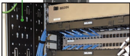
Lacing Panel shown in cabinet
