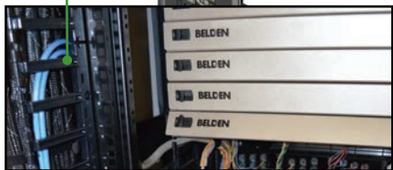
Vertical Manager shown in cabinet
